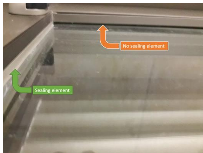
Figure 8 – Lack of sealing element
